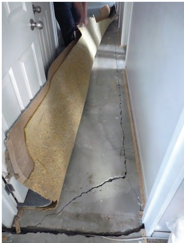
Slab cracking after the Canterbury earthquakes
